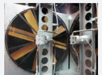
Hydraulic oil cooling fan
