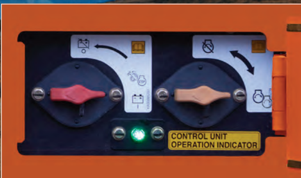
Battery & starter isolation switches
